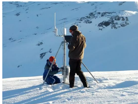
Redundant Radio System (sub 1-GHz, monitoring natural hazards)
