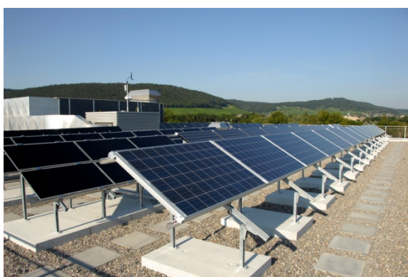
Figure 2: The EKZ Outdoor Test Reference Installation in Zurich is equipped with about 100 PV modules out of five different technologies (see Table 1). The modules of each technology are grid connected by a typical 3 kW inverter and one PV module is independently IV curve tested each minute. All measurement results are recorded in a database structure and further on analysed [2]. All modules are periodically tested by the SMFB.
